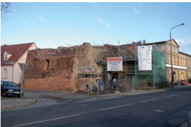
Fig. 32—34: Peitz. Malzhaus bastion. Partly open structure, not hitherto receiving building maintenance.
