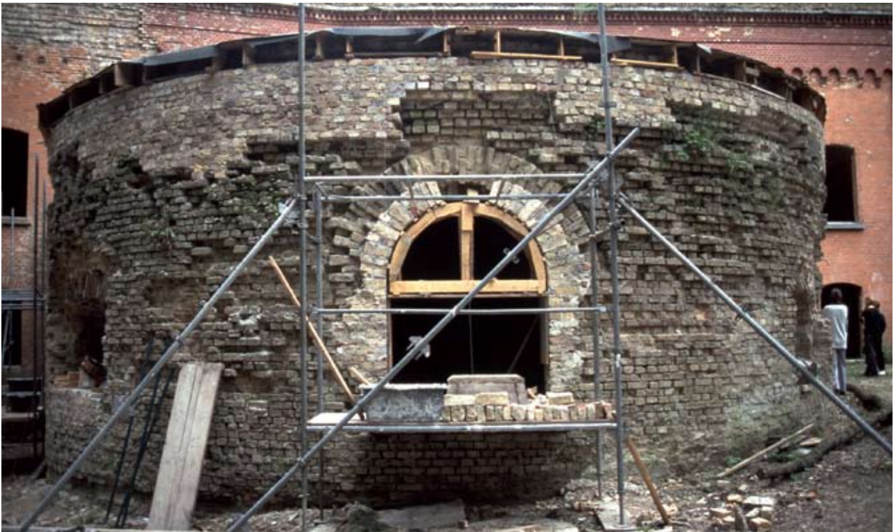
Fig. 31: Berlin-Spandau. Fort Hahneberg. Remedial work on the gorge caponnier. Basic use of any kind will require stable, secure structures.
